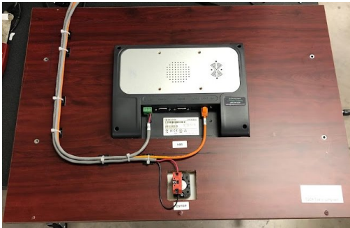
(a) HMI Wiring on Podium
